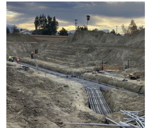
San Jacinto Valley Groundwater Treatment Facility Phase I
